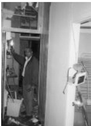
Ghanshyam surveys the damage.
